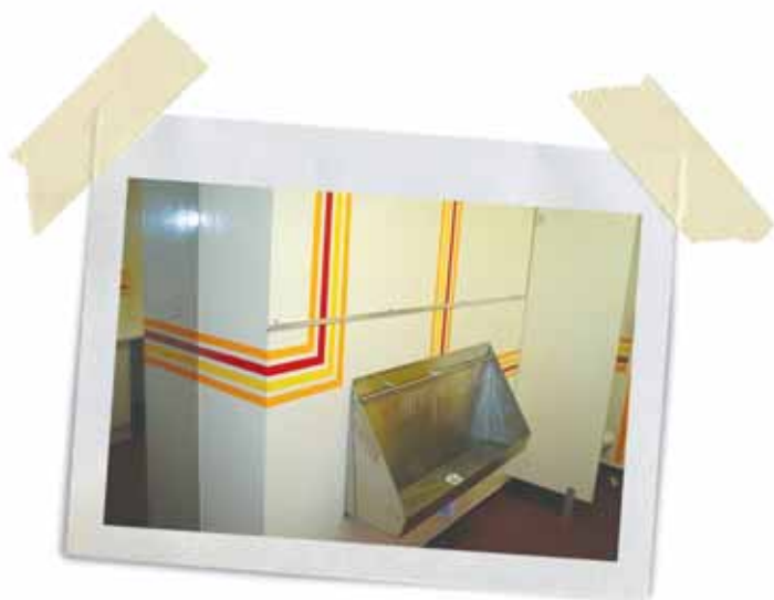
▲ Above trough urinals should be avoided
