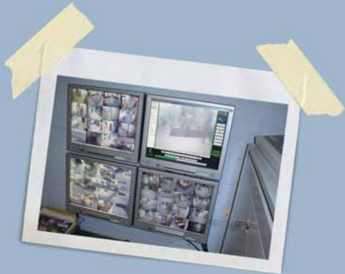
▲ Above CCTV should be avoided
